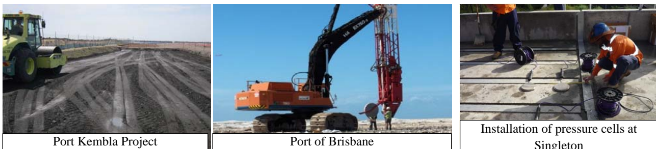
Fig 3. Compaction Field Trial at Port Kembla Reclamation Project, vertical drains installation in Port of Brisbane and field monitoring of track behaviour at Singleton.
